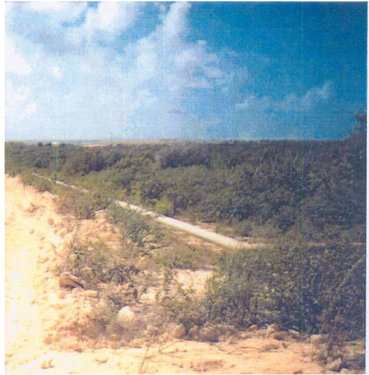
Photograph 3: Power Station fuel pipeline and ShellIDelta access road
